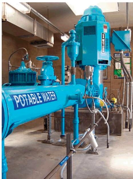
City of Roseville ASR well
