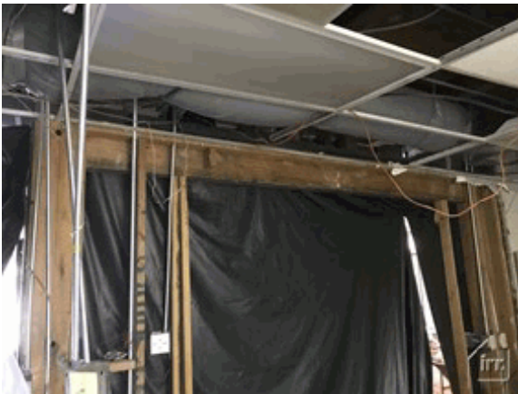
Interior –structural issues with the addition
