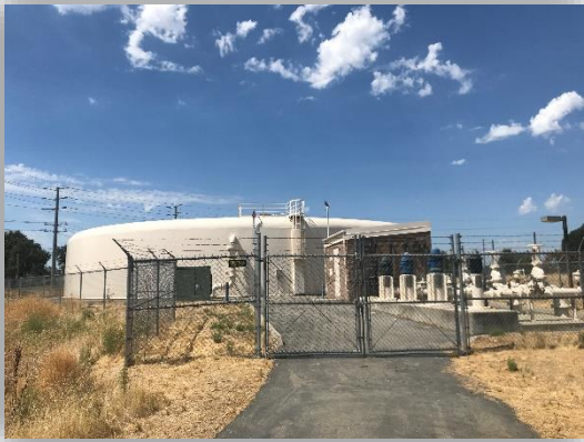
North Zone Pump Station
