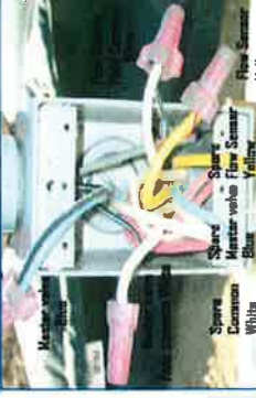
Master valve wiring installed correctly.
