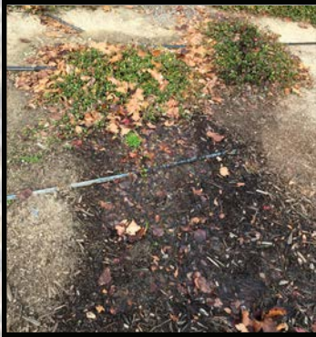
Failed subsurface drip irrigation
