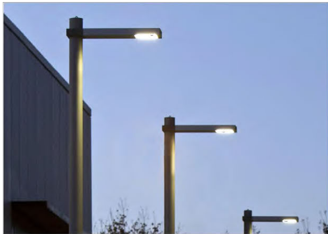
ROADWAY LIGHT FIXTURES
