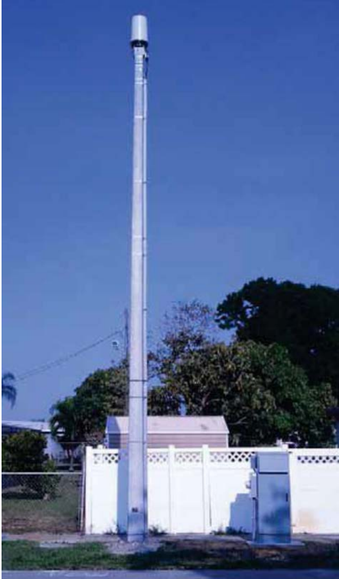
Figure 1: Example of Small Cell application
