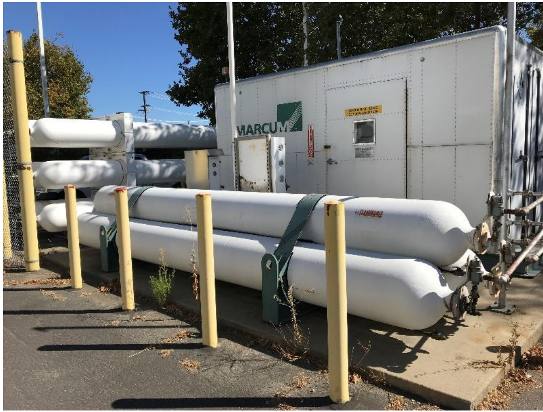
Site 1. Storage Vessels and Gas Compression Skid
