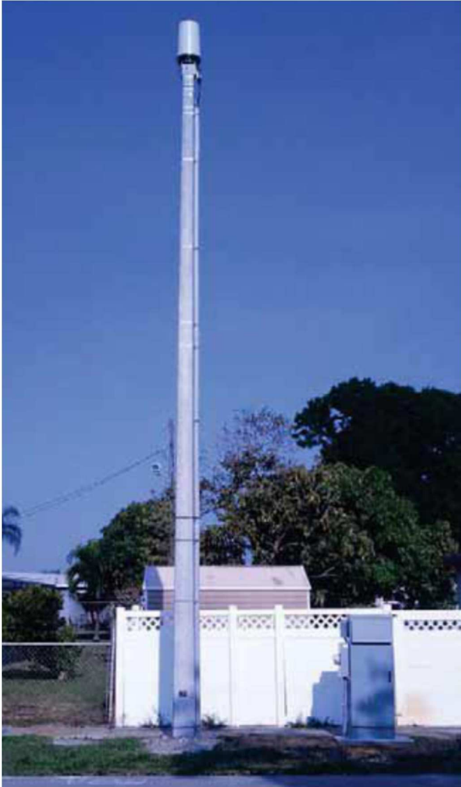
Figure 1: Example of Small Cell application
